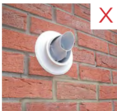
Poorly considered building services
